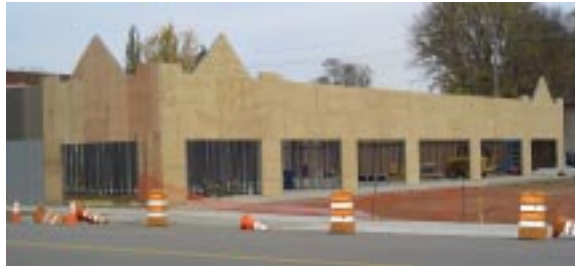
Progress continues in downtown Marshall on the building to be occupied by Movie Gallery, changing the face of the central business district. Movie Gallery expects to open in mid- December.
